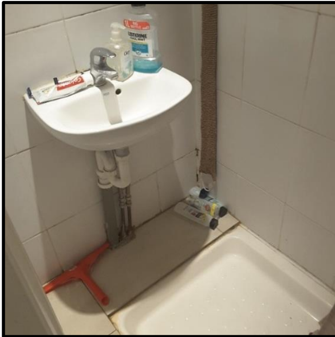
Wash hand basin located inappropriately within shower cubicle.
